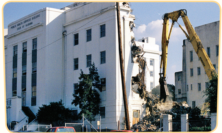
Earl Langley of the Office of EMS and Trauma photographed the building's demolition during November.
